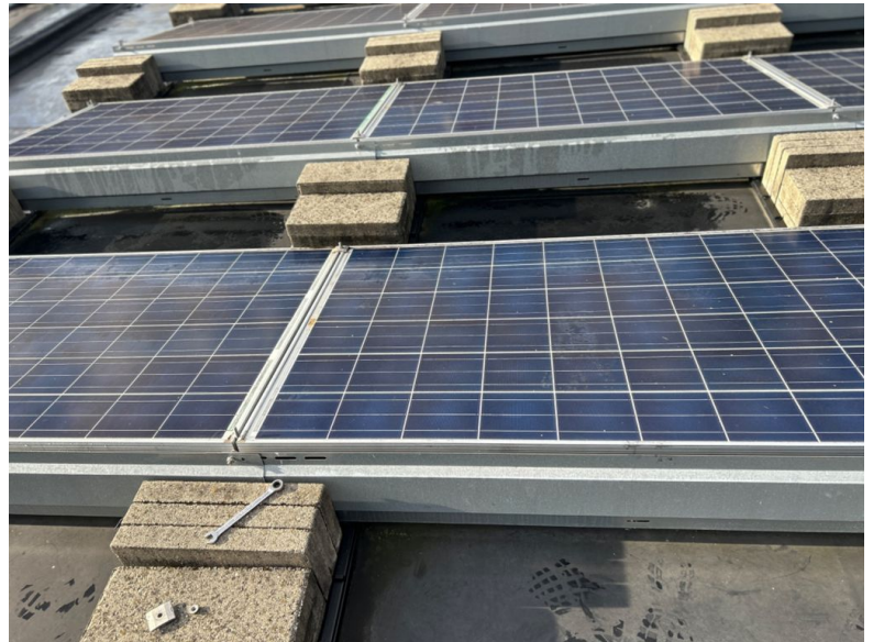
Pictures taken before repairs made._6
