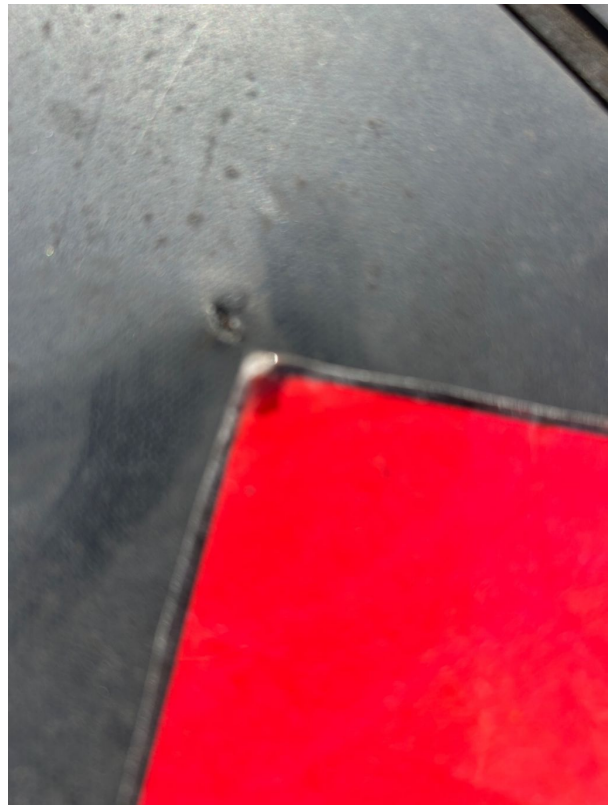
Pictures taken before repairs made._2
