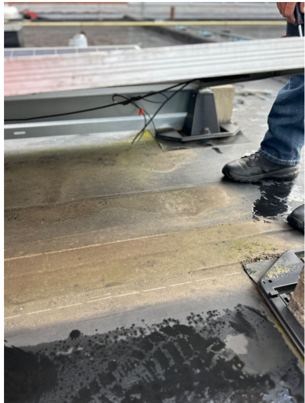
Pictures taken before repairs made._4
