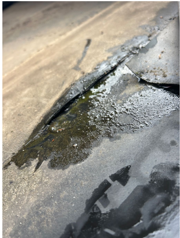
Pictures taken before repairs made._8
