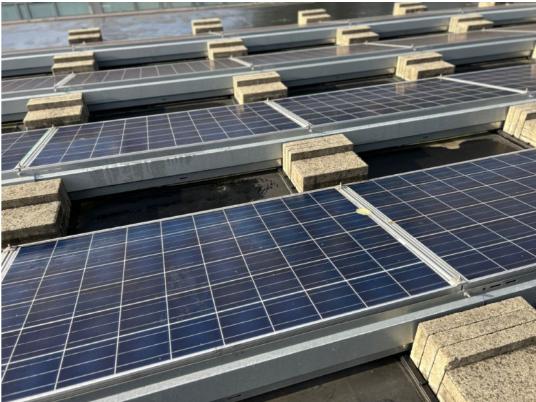
Pictures taken before repairs made._7
