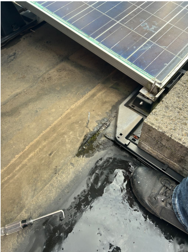
Pictures taken before repairs made._9
