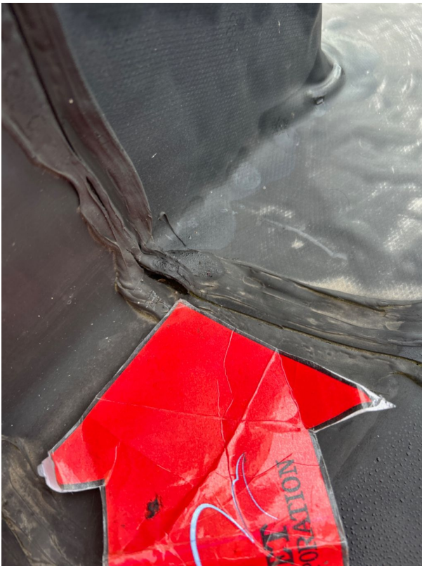
Pictures taken before repairs made._3
