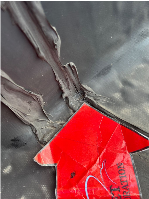
Pictures taken before repairs made._5
